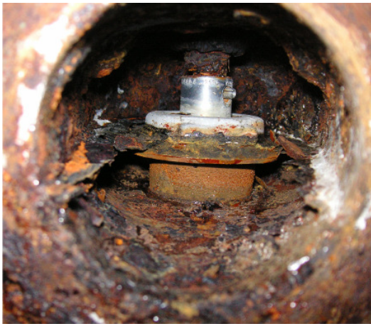
Figure 17.3.4-1: Symptom 12 - Strong corrosion in a safety valve
