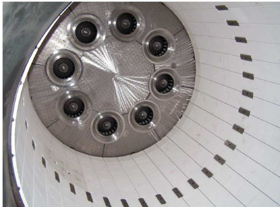
Silo - Combustion Chamber View to Flame Tube
