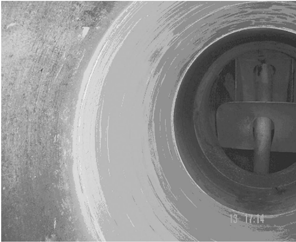
Fig. 1 Structural Liner in Raw Water System
